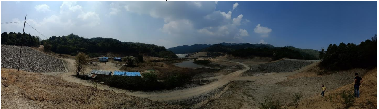
Figure 3-21: Undergoing development of Dhap as a Recharge Lake near to Chisapani in Shivapuri National Park
