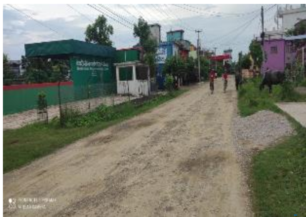
Condition of the road in Ward on 7
