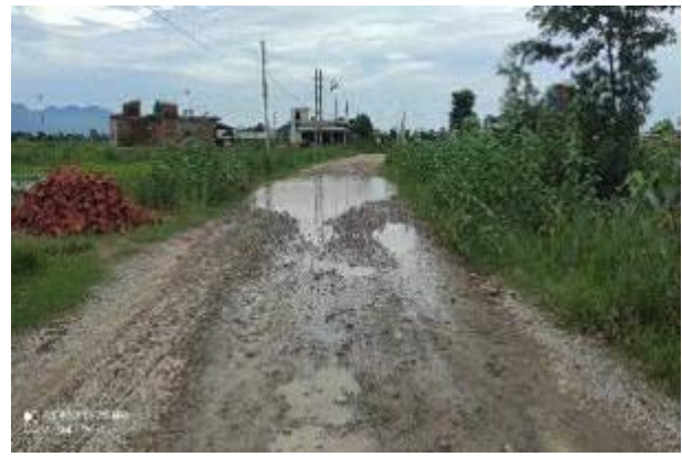
Condition of existing road
