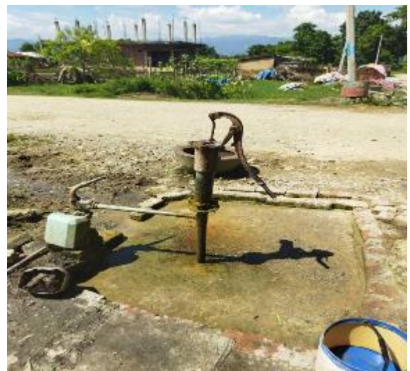
Hand pump near road RoW
