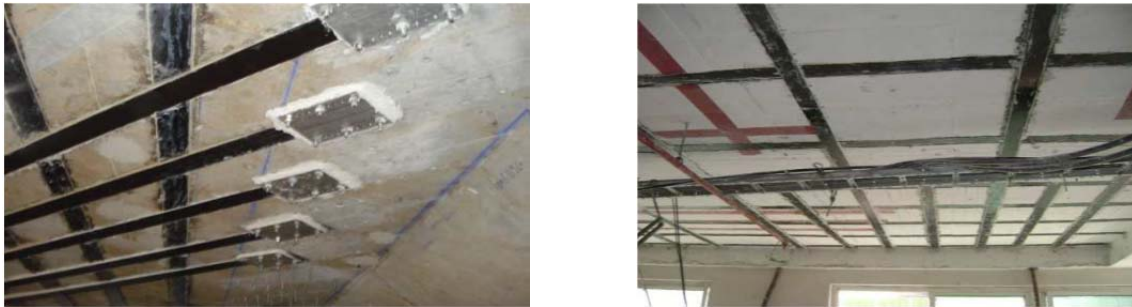
Figure 9-2 Use of Laminates in for strengthening of slabs in a bridge and a building (Source: Hari Darshan Shrestha)
