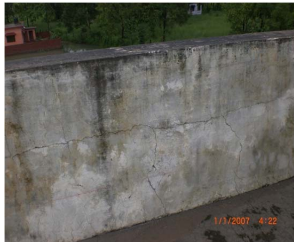
Figure B-20: Crack at Parapet wall
