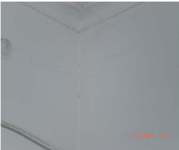
Figure B-19: Crack at wall
