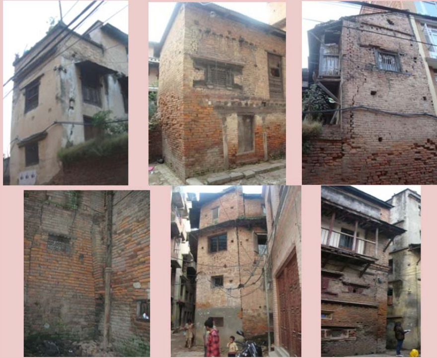
Cracks seen at corners in old buildings in Lalitpur, Nepal Photo: Ar. Anjali Manandbar
