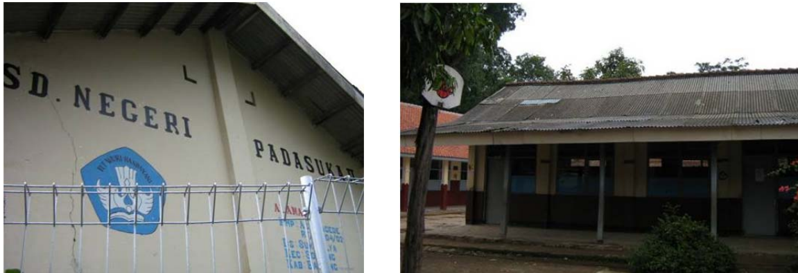
Figure B- 1: Layouts and Existing Conditions of SDN Padasuka II Prior to Retrofitting
