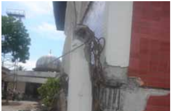
Soft Ground Storey
