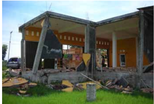
Weak Beam- column Joint
