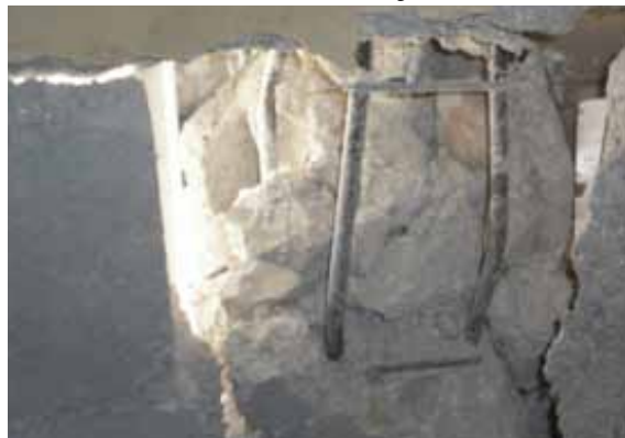
Due to confinement
