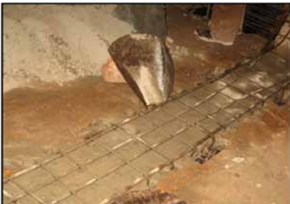
Figure 6.14 Beam Jacket (Source: MRB & Associates)
