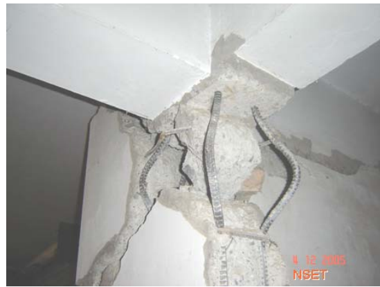
Photo 22: Buckling of column bars
