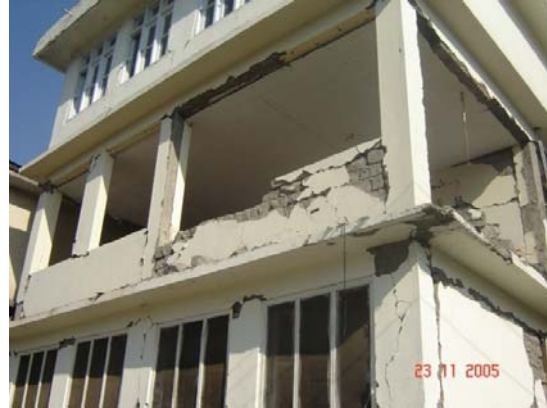
Photo 24: Extreme Damage to Infill wall
