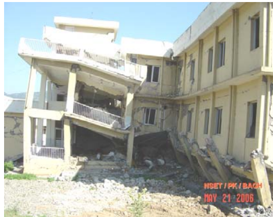
Photo 18: Earthquake damage due to soft story
