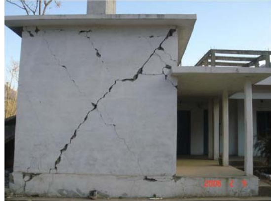
Photo 8: Diagonal cracking of solid wall
