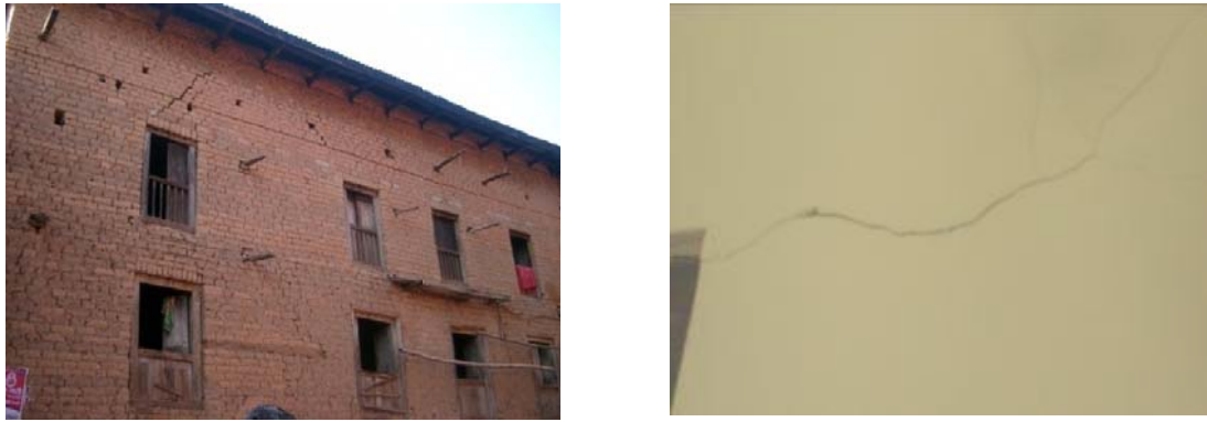
Fig 2.11 Problem due to Crack in Brick Wall
