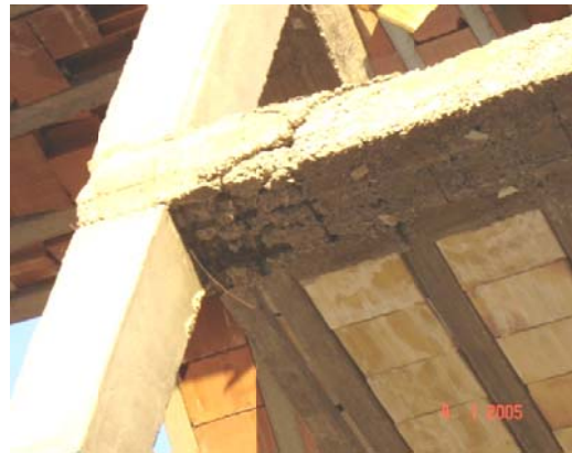
Photo 20: Shear crack in beam near to support
