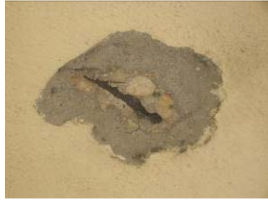
Fig 2.9 (b) Rusting of Steel Bar
