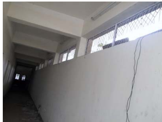
Fig 2.13 (b) Ventilator Attached to Frame
