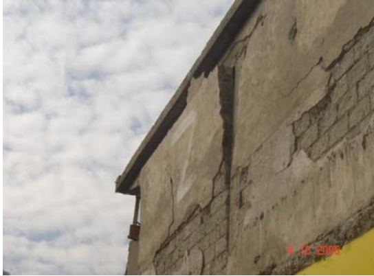
Photo 23: Moderate-Heavy Damage to Infill wall
