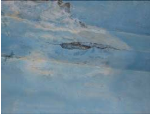
Fig 2.9 (a) Delamination due to Seepage of Water
