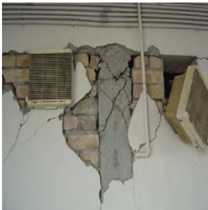
Photo 21: Shear crack in column
