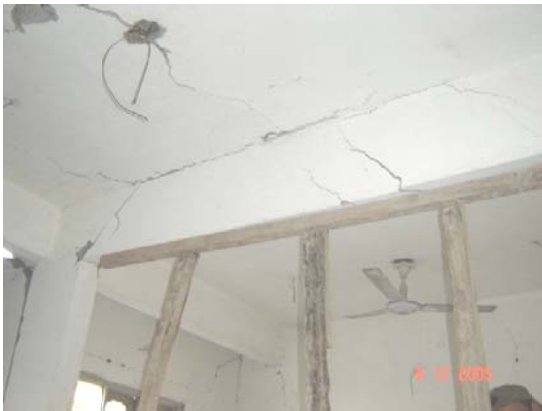
Photo 19: Shear cracks in beam near to support and at mid span
