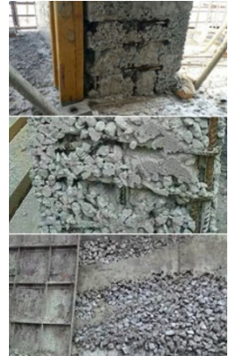
Figure 14: - Pouring concrete from a greater height causes segregation.
