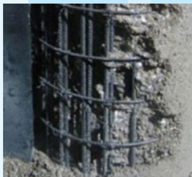
Figure 18: - Substantial gap, hole, or defect found during inspection in concrete.
