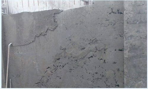
Figure 16: - Honeycomb seen in concrete without the use of vibrator.
