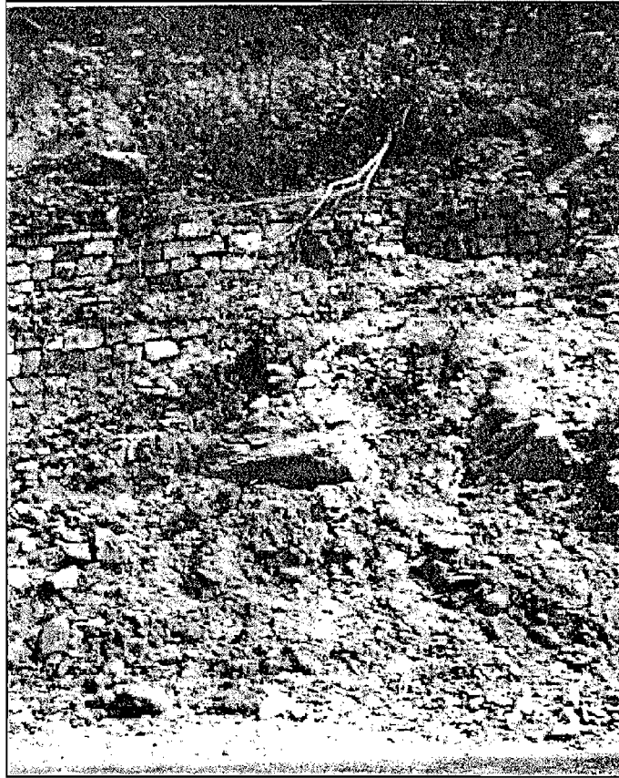
Plate 9: Concrete masonry wall would have been appropriate here
