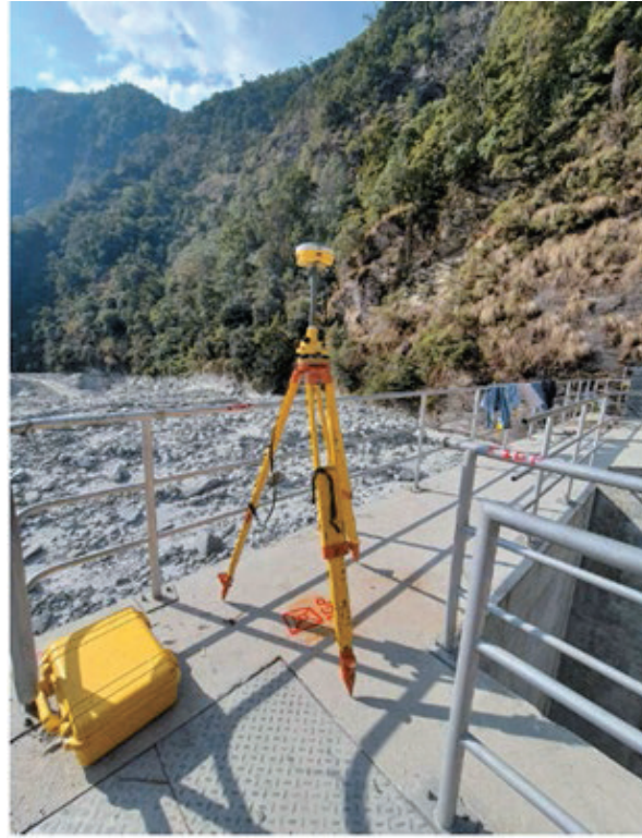
Survey work is carried out in the debris-strewn headworks area (photo by Explorer Geophysical Consultants Pvt. Ltd).
