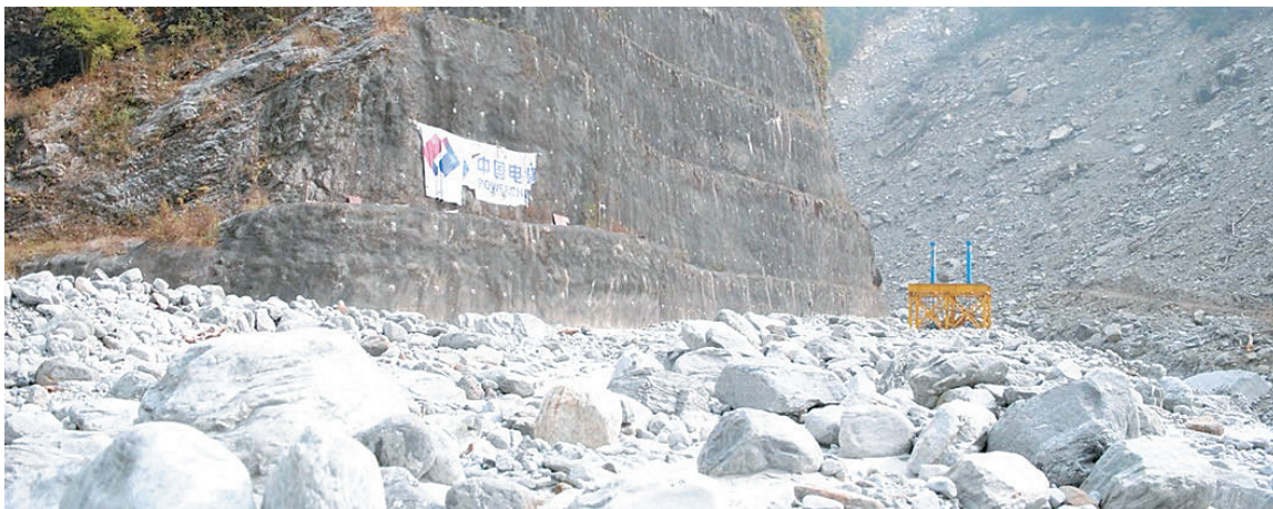
Pre-disaster (above) and post-disaster condition (below) of Melamchi headworks (photo by TA team)
