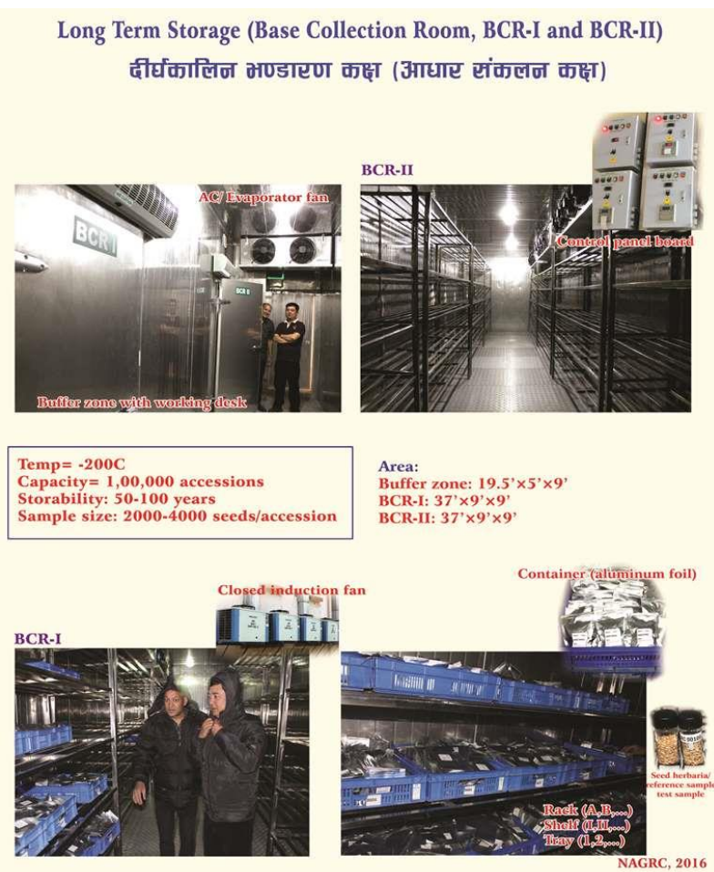
Figure 8. Functional parts, process and details of long term storage room.
