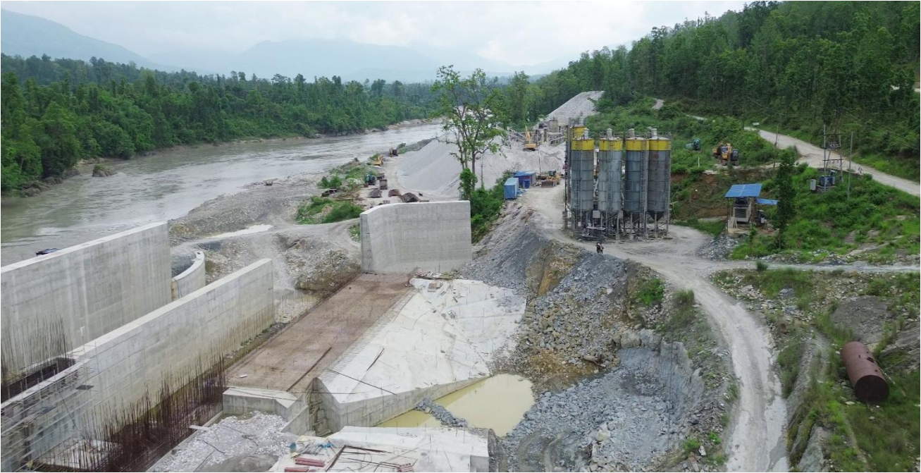
Figure 5 Intake Gravel Trap
