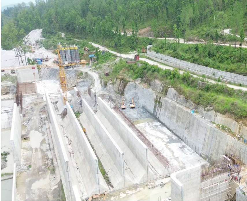
Headworks- Settling Basin
