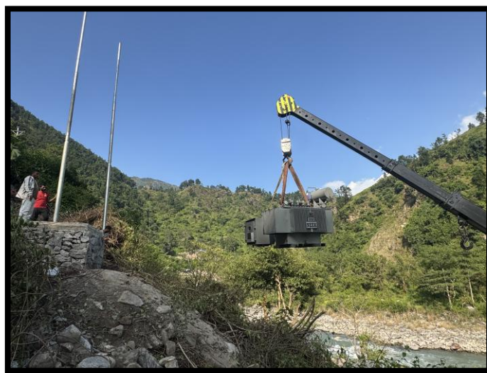
Transformer Installation at Crusher Site for Construction Power
