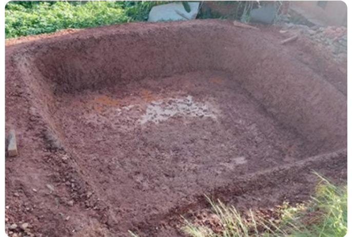
Figure 12: Pond for water recharge
