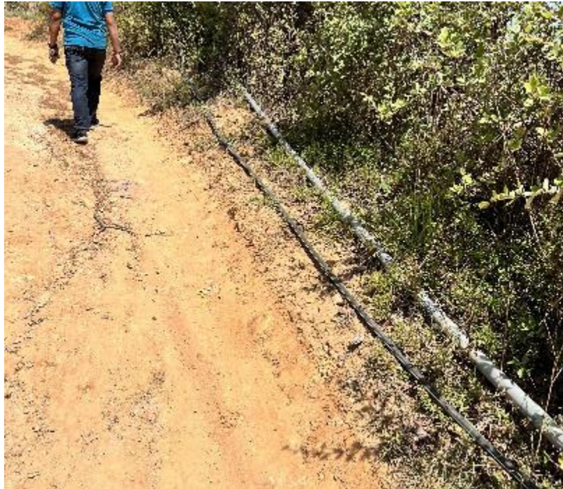
Steel pipe used for drinking water supply that needs relocation during road construction
