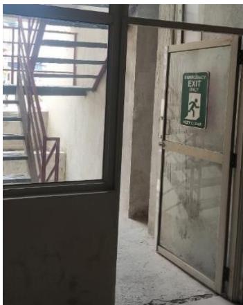
Fire Escape stair with exit signage
