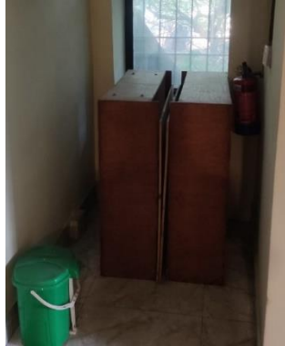
Fire Extinguisher obstructed with cabinet in corridor
