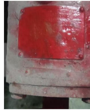
Fire pump information tag being painted over
