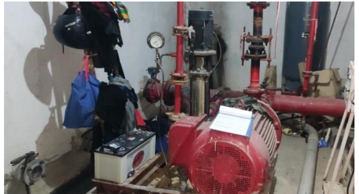
Congested fire pump room with extreme storage of waste materials
