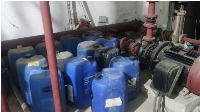
Fire pump room congested because of storage of empty containers
