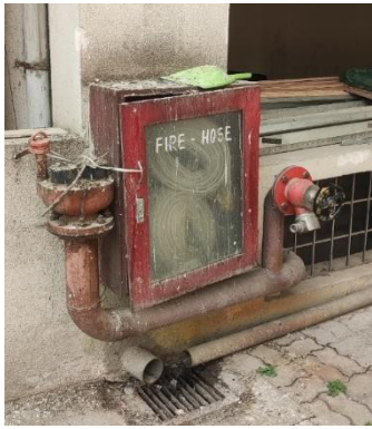
Outdoor valves and cabinet in bad condition due to lack of maintenance
