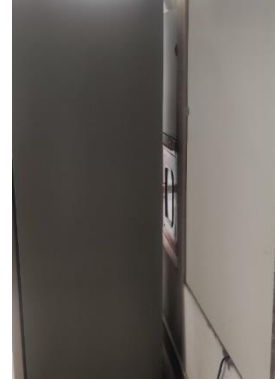
Fire hose cabinet blocked by personal item (fridge) installed in front of cabinet
