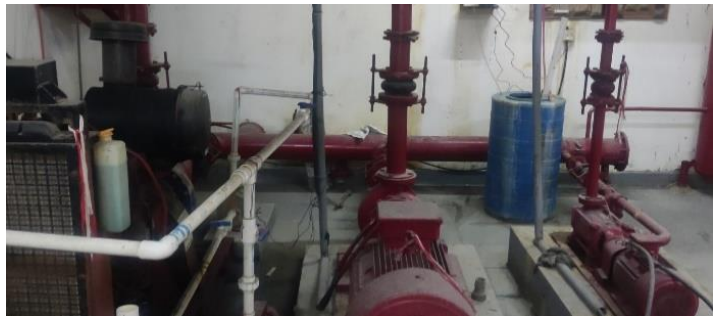
Clean and easily accessible fire pump room
