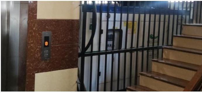
Generator installed next to open evacuation staircase
