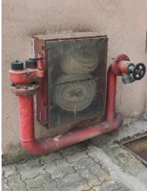
Poorly maintained valves and cabinets
