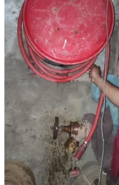
Leakage in Fire Hose Reel pipe
