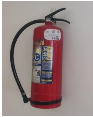
Expired Fire Extinguisher still installed
