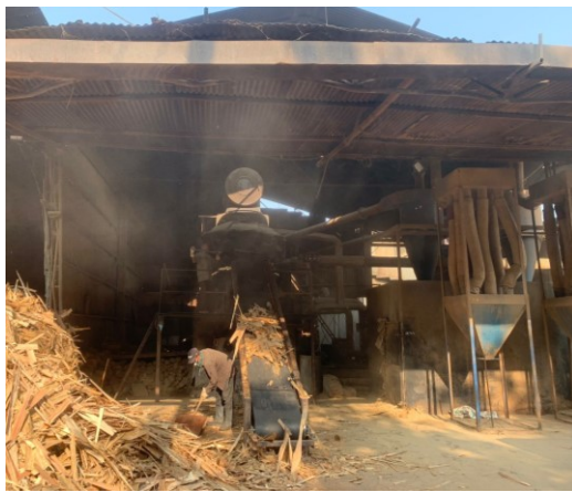
Saw dust & cut pieces used in Boiler as fuel
