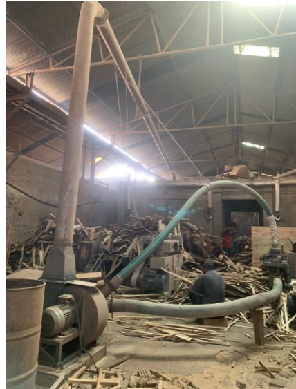
Dust collection system
