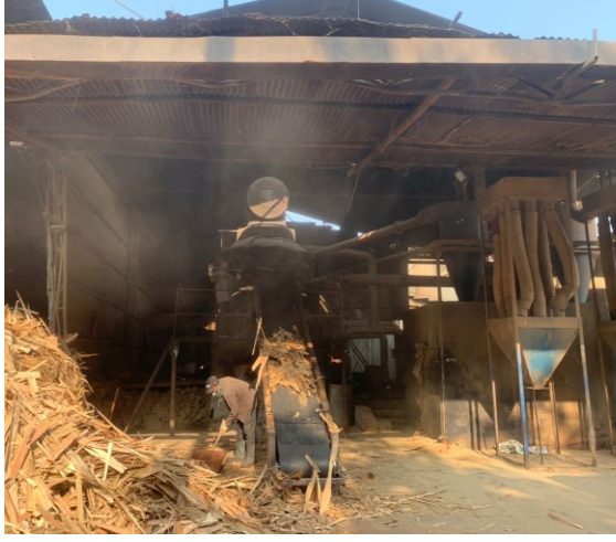
Boiler section with dust collector and bag house
