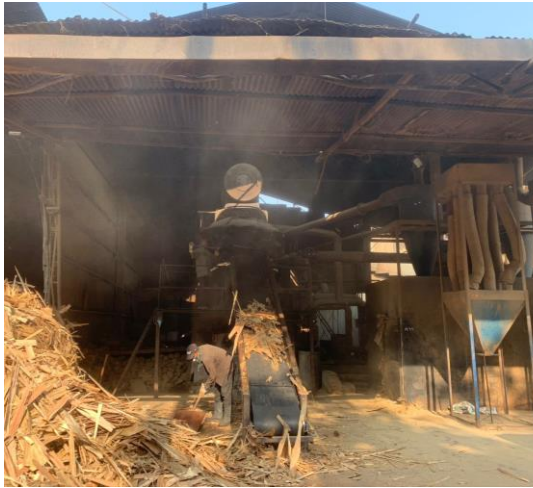
Boiler with dust collector and bag house
