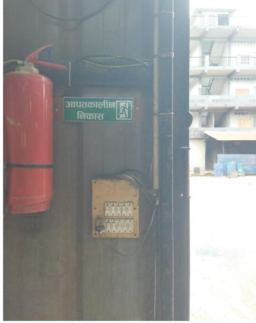
Fire Extinguisher and Emergency Exit
