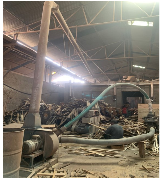
Dust collection system
