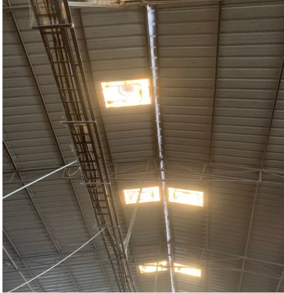
Rooftop natural ventilation
