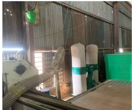
Baghouse installed at door designing section
