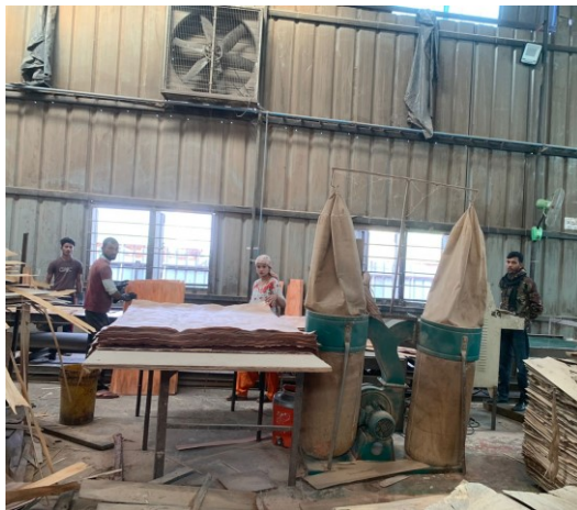
Baghouse for collecting sawdust
