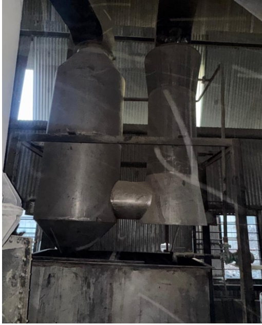
Wet scrubber and cyclone installed in boiler
