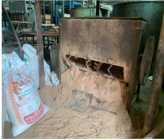
Saw dust collected from dust collector for reusing as fuel in Boiler
