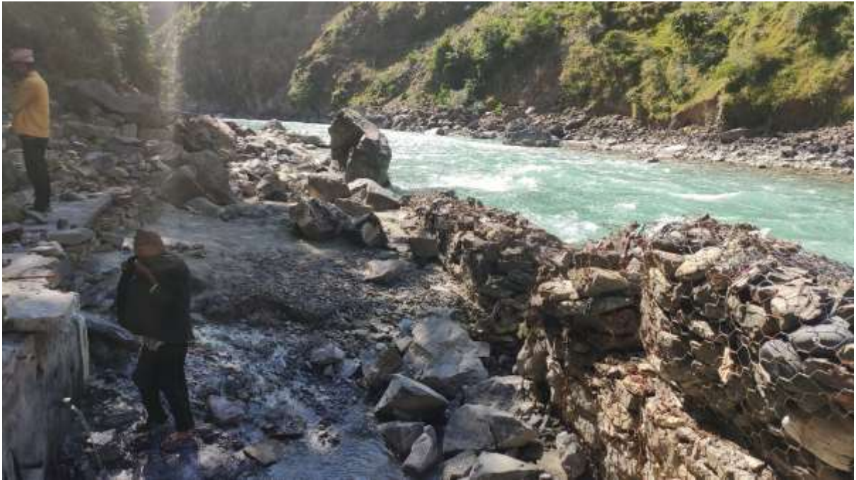
Photograph 5.72: Hot water spring and the protection work done at the Agra Tatopani
