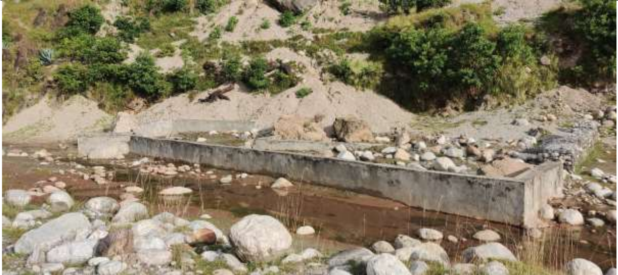
Photograph 5.40: Protection work done to safeguard the hot water spring at the Sisne Tatopani
