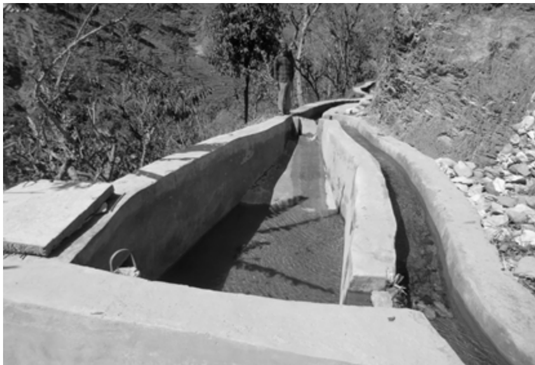
Figure 5: The forebay of micro-hydro project in the main canal of irrigation scheme
