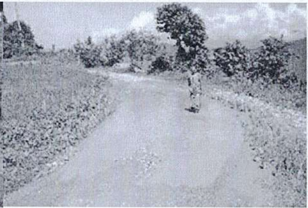
Water stagnation in depressed road surface
