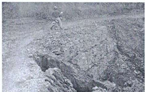
Gully formation in the road shoulder
