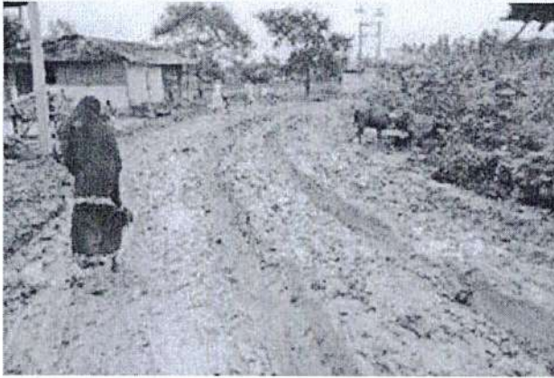
Rut formation in waterlogged areas
