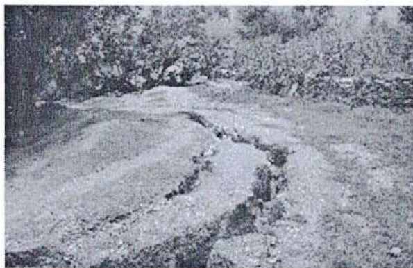
Erosion of the road surface
