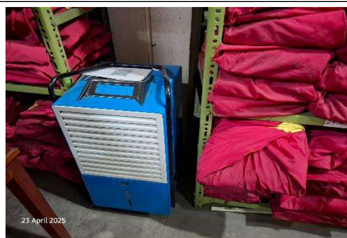
Dehumidifiers provided in archival storage room.
