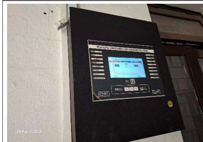
Fire detection panel system.
