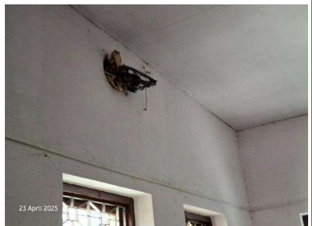
Damaged exhaust fan.
