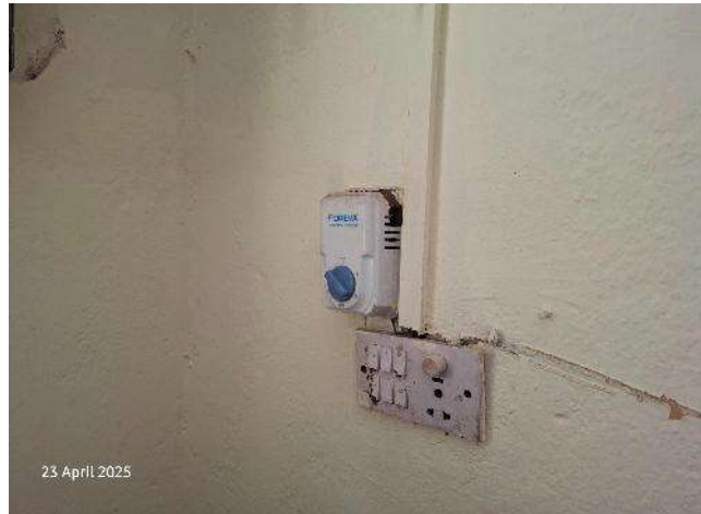
Damaged electrical switches.
