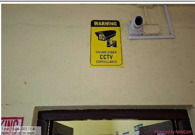
CCTV installed across the building and rooms.
