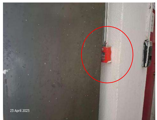
Emergency alarm break glass manual call point blocked.
