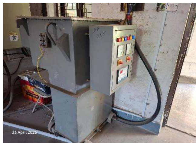
Batteries were stored near electrical panels.
