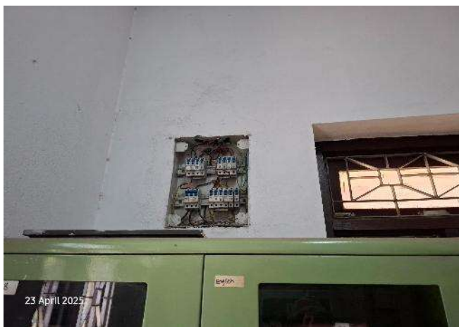
Electrical panel left uncovered.
