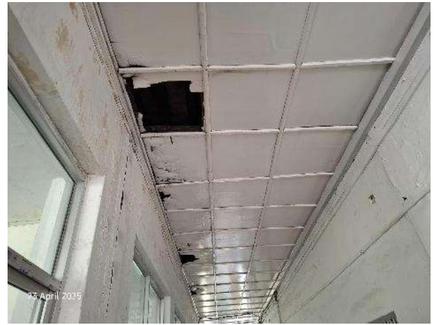
Several ceiling panels found damaged.
