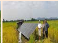
Photo 2: Diesel replaced after Solar PV pumping system
