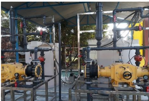
Chlorine Dosing System
