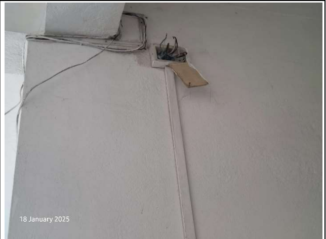
Damaged and exposed electrical cables.
