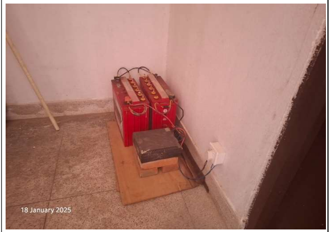
Battery charging station at corner of corridor without any safety precaution.
