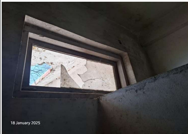
Damaged window's glasses of toilet.
