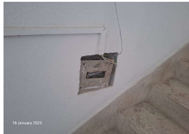
Damaged electrical panel.
