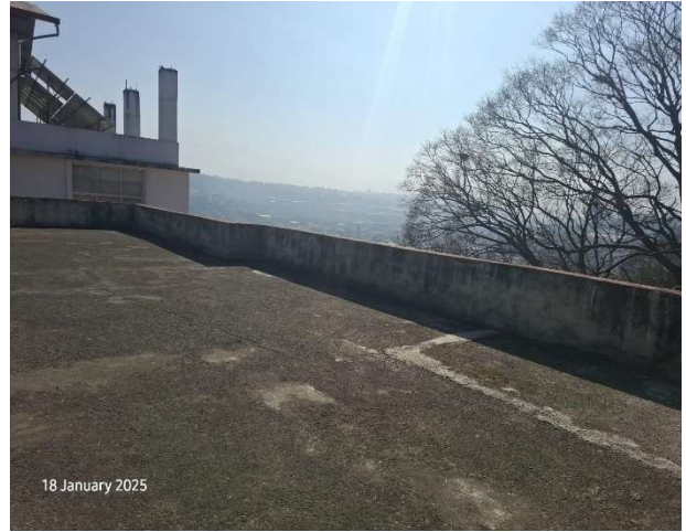
Height of parapet wall is short.
