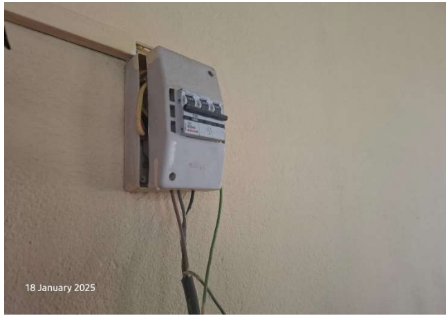
Electrical switches board left opened.
