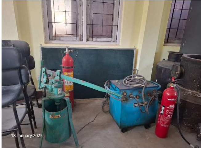
Fire extinguishers without regular inspection.
