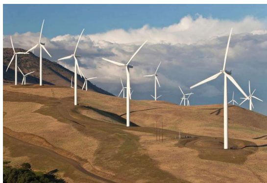
(a) Horizontal Axis wind turbine
